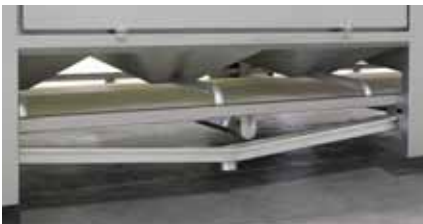
Washing system drainage.
