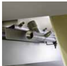
Conveyor belt washing system.
